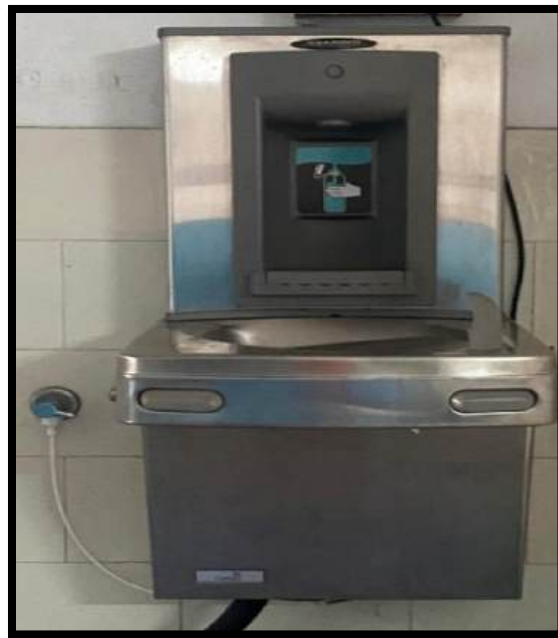
Drinking water purification system
