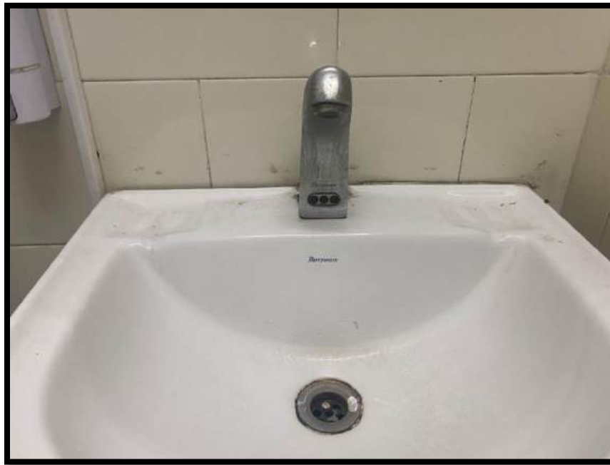
Water efficient fixtures in bathrooms of Management House, IEM Campus
