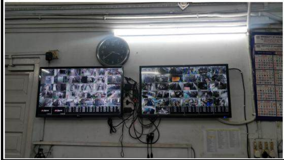
Campus Surveillance through CCTV Cameras
