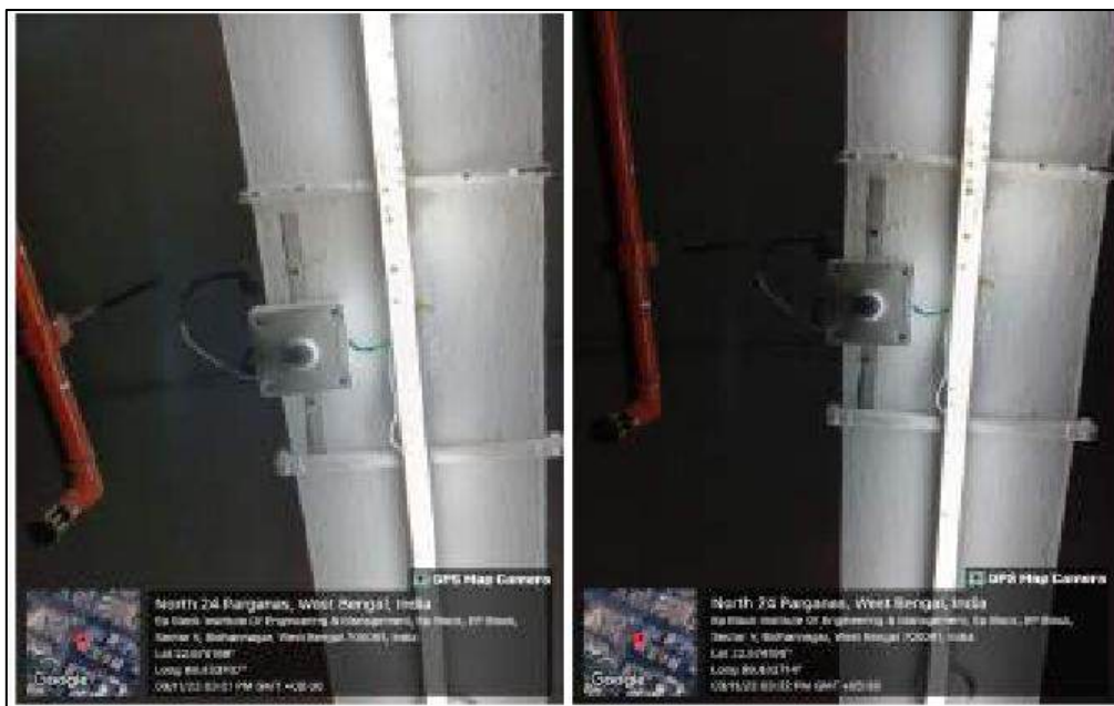
Sensor-based energy conservation system
