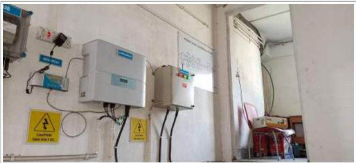
Solar Grid box
