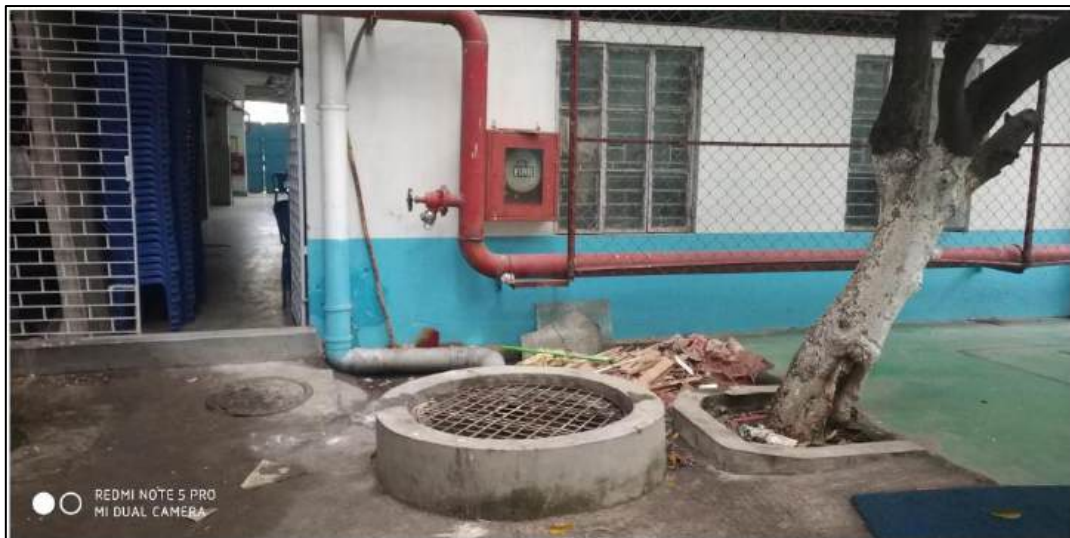
Rain Water Harvesting
