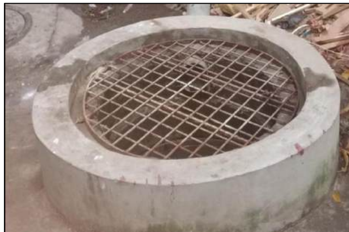
Rain Water Harvesting
