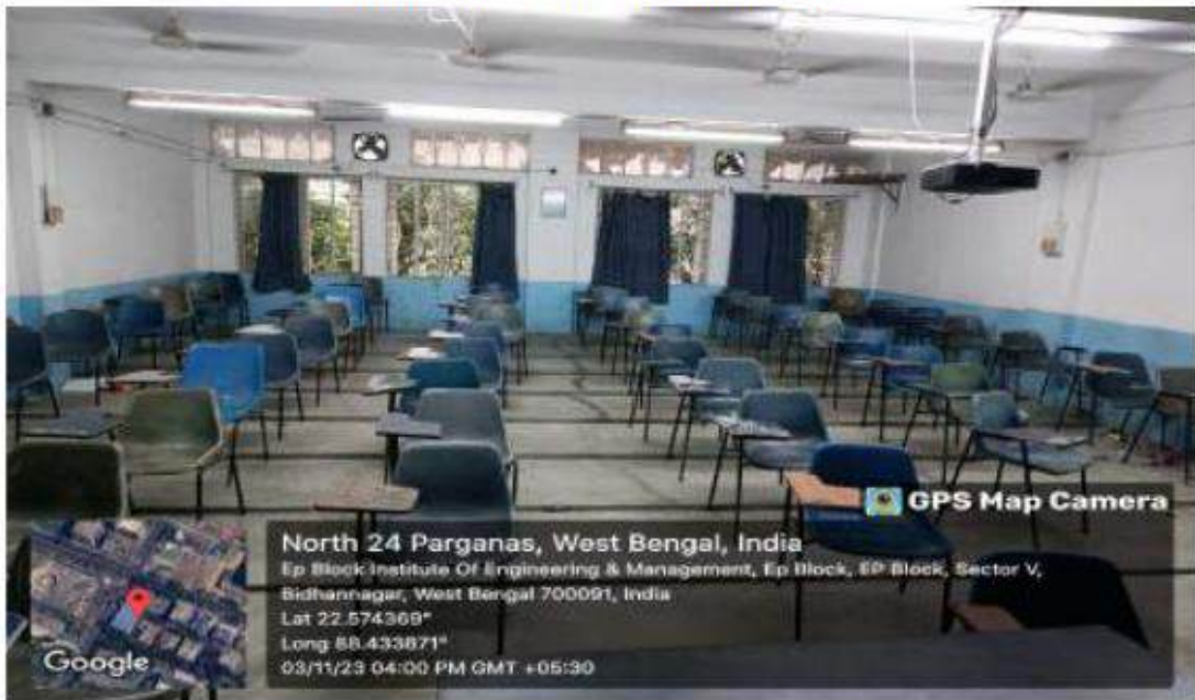
Photo: LED Tube Lights in Classrooms
