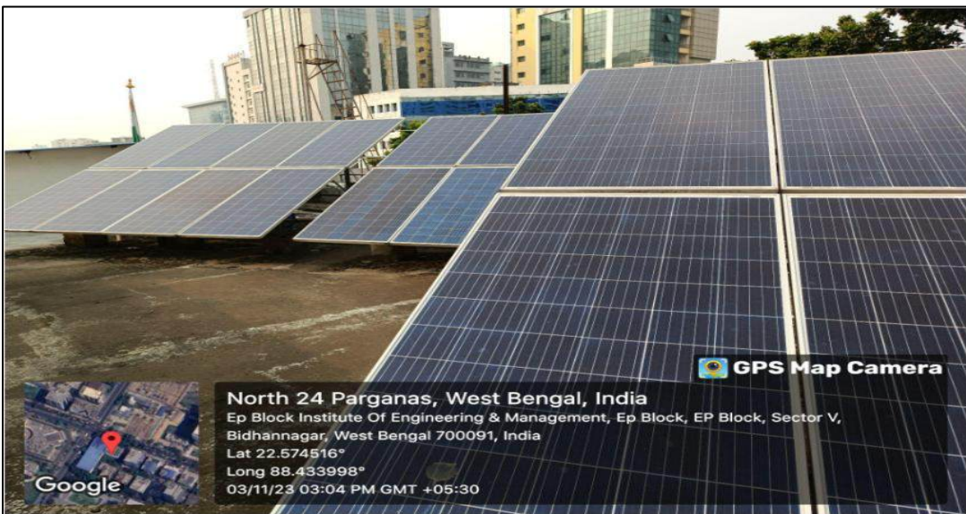
UEM Kolkata leads sustainable innovation with extensive solar panels harnessing renewable energy across its campus rooftops and facilities.
