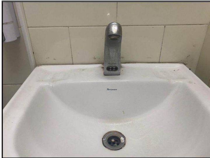
Water efficient fixtures in bathrooms of Management House, IEM Campus
