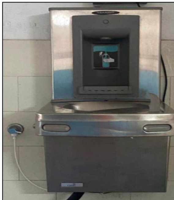
Drinking water purification system
