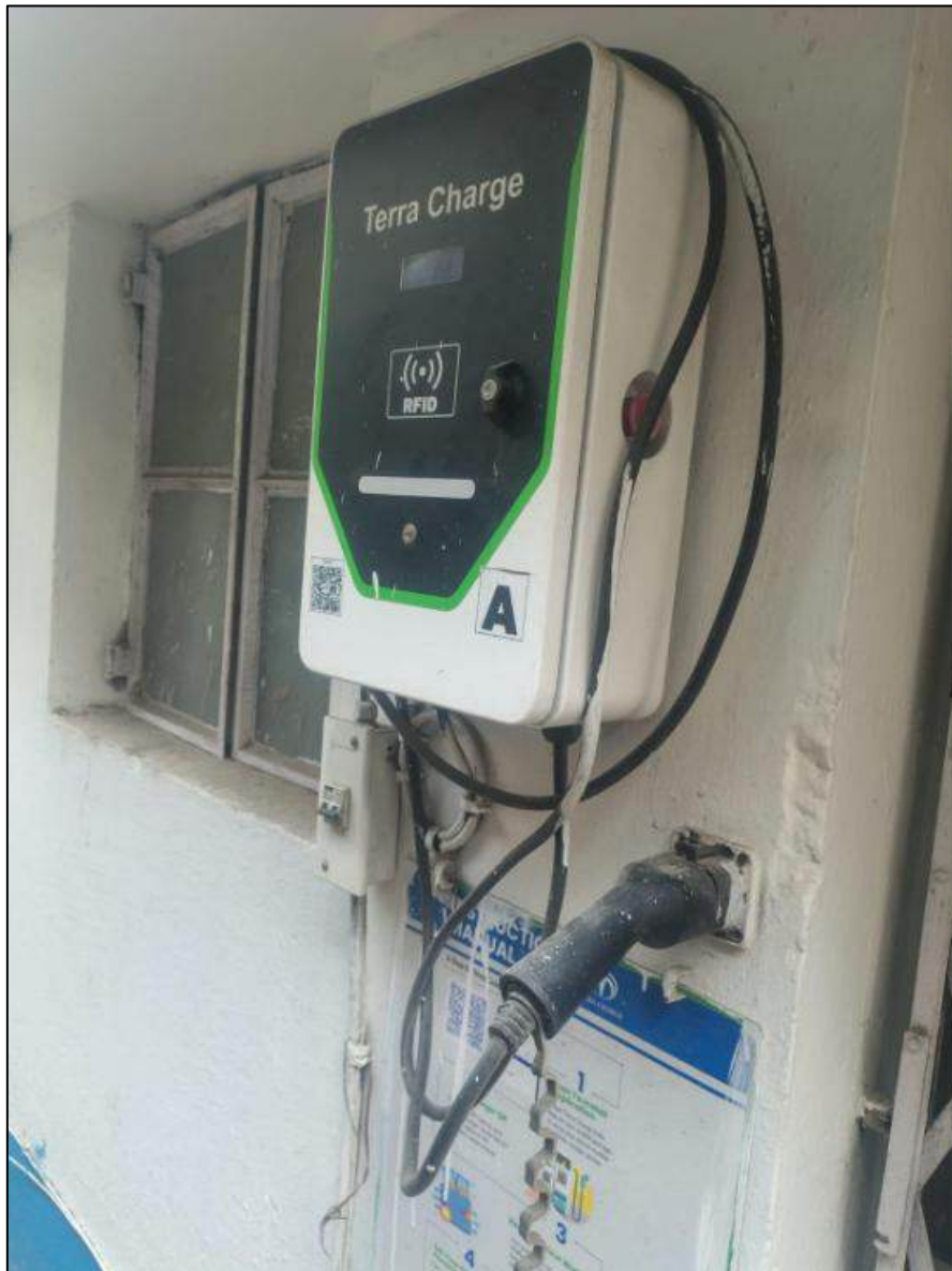
EV charging points installed to promote electric mobility on campus
