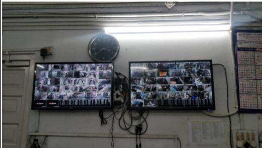
Campus Surveillance through CCTV Cameras
